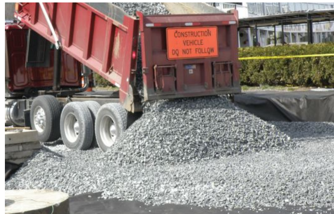
In reservoir course placement, the 100% fractured stone courses are critical to stormwater storage, structural support, and in-place density of the porous asphalt. CREDIT: BARTON & LOGUIDICE, D.P.C.
