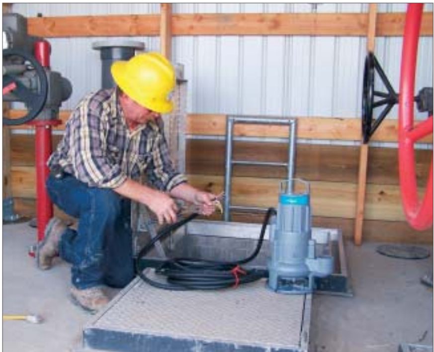
One of the ITT Flygt leachate transfer pumps being prepped for installation. The volume of flow is metered to ensure compliance.
