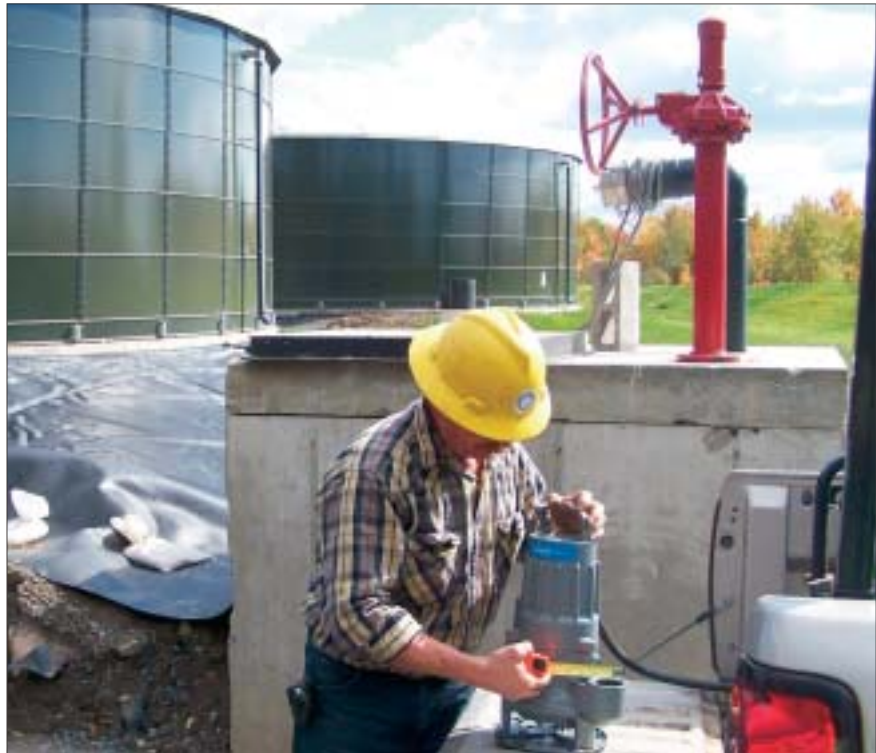
One of the ITT Flygt pumps that transfer collected leachate to the 1.3-MG tanks in the background is being prepared. Tanker trucks will off-load and haul the leachate to a wastewater treatment plant.
